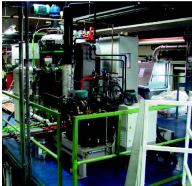
The piston-dosing high pressure metering unit is usually located over the spray booth.
